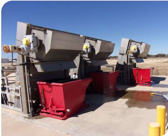
Typical plastic pellet discharge setup using a lined dumpster
